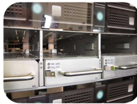
Battery Backup Unit
